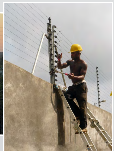
Petro Chemical Plant, Nigeria
