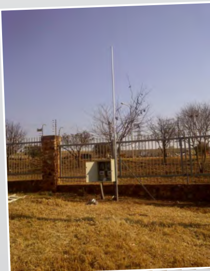
Wireless Repeater Station
