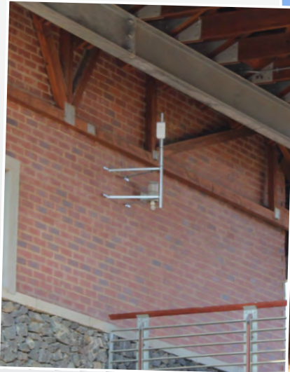
Wireless Transceiver Installation
