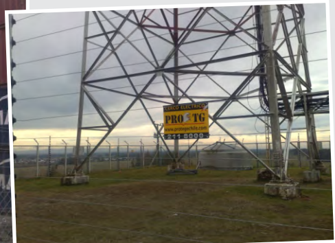
Power Station, Chile
