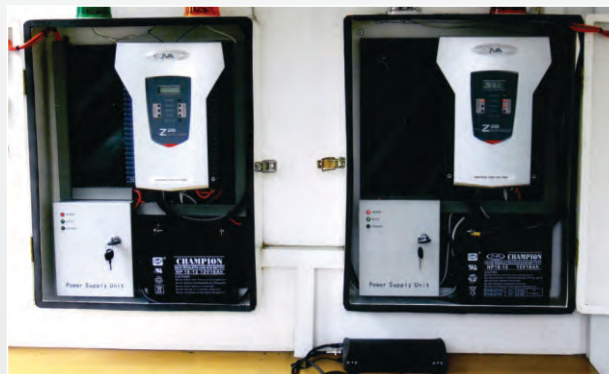
Synchronized System – Internal View
