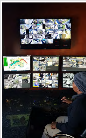
Housing Estate, Control Rooms
