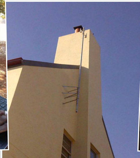
Wireless Transceiver at Control Room
